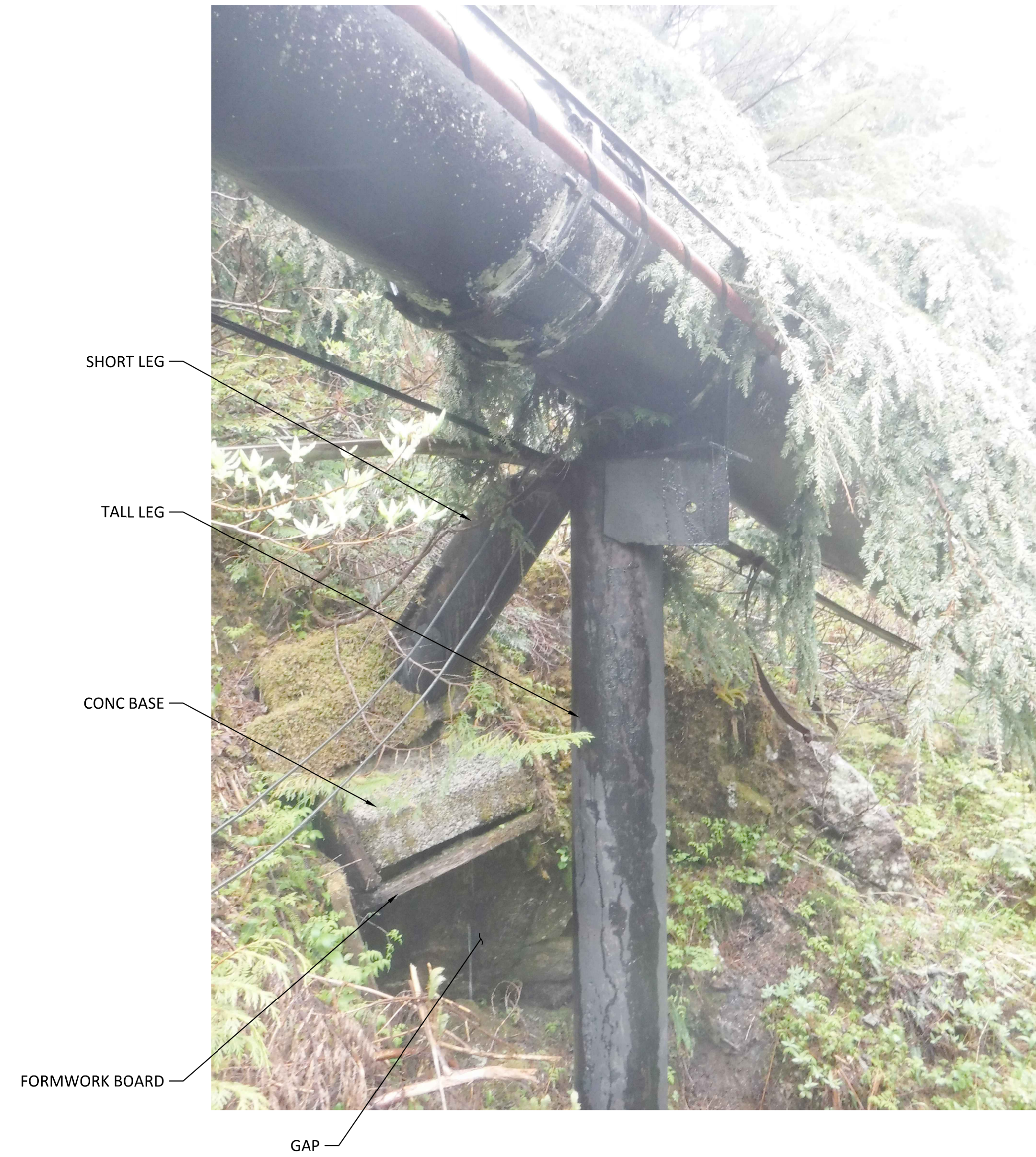
PHOTO - SUPPORT @ COUPLING NO. 105
