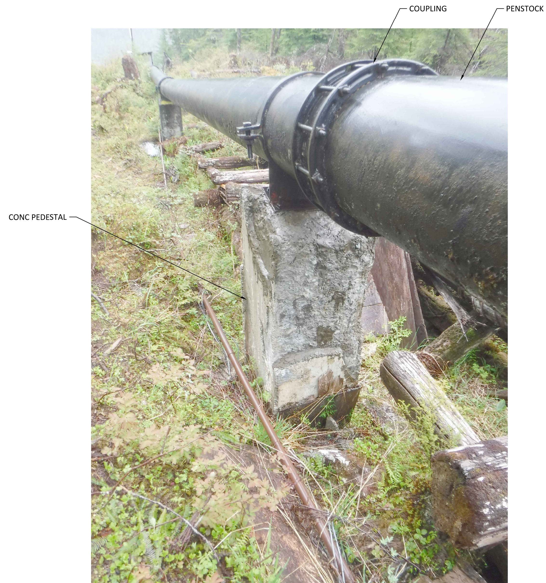
PHOTO - SUPPORT @ COUPLING NO. 68
