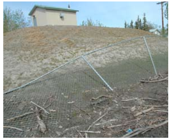
Sewage pumping station elevated on mound—Fort Yukon
