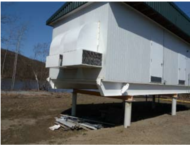
Adequate elevation protects power generator—Sleetmute
