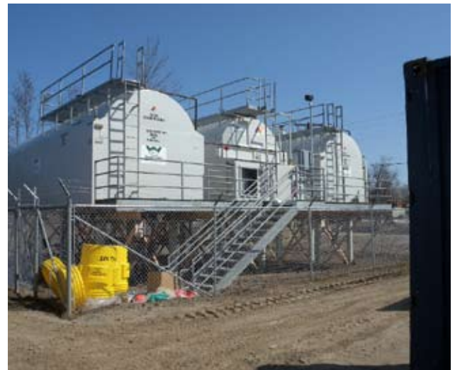
Fuel tanks supported above flood level—Sleetmute
