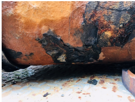
Severely corroded pipe removed from Sandy Beach area in 2018.
